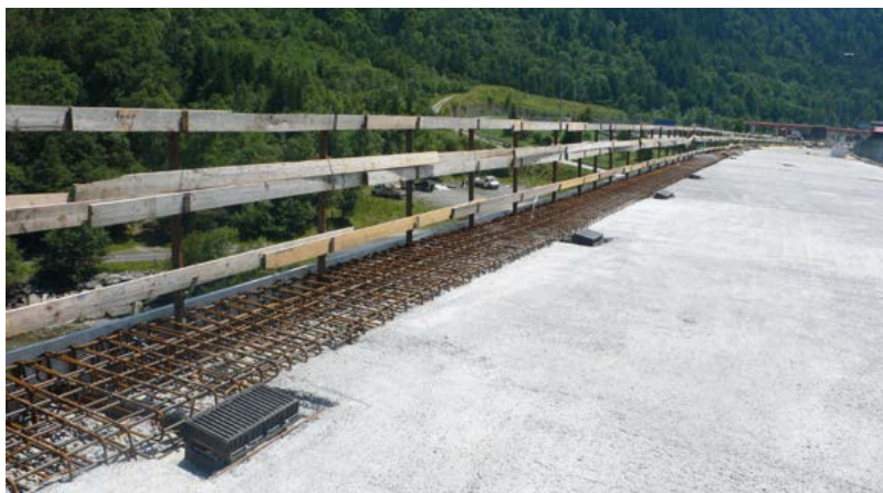
Bridgedrain - Cuneo (CN)
